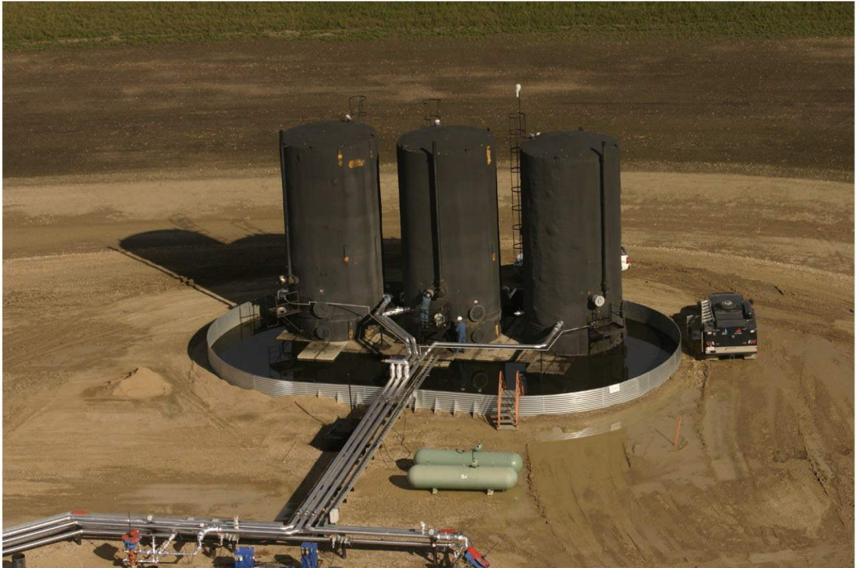
Containing 3; 1,000 Bbl tanks
