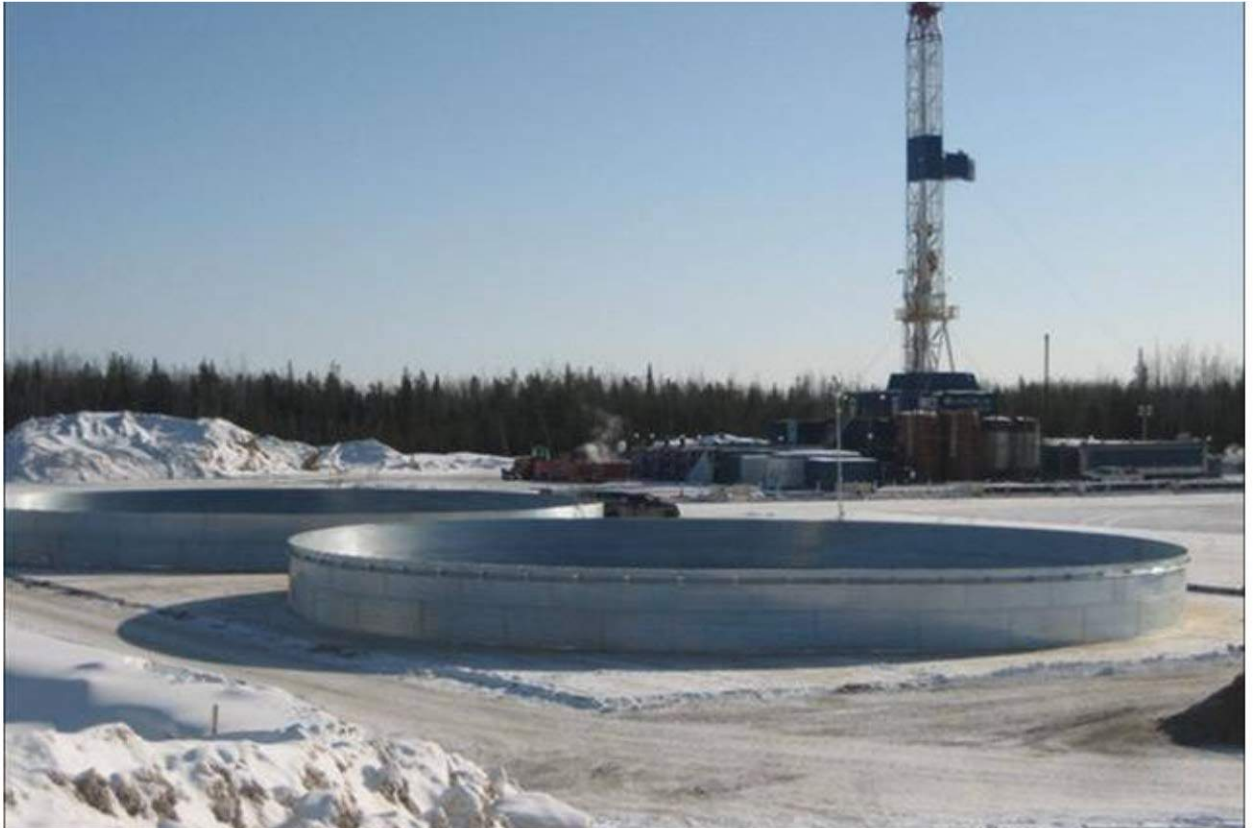
Frac Water Tank 96' Diameter x 7' 4" High Capacity: 1,489 m 3 Ramshorn, B.C.
